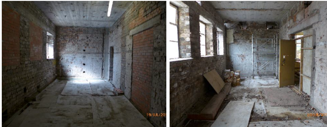
Upper Ground Floor - Existing ladies and Gents WCs next to main stair.
