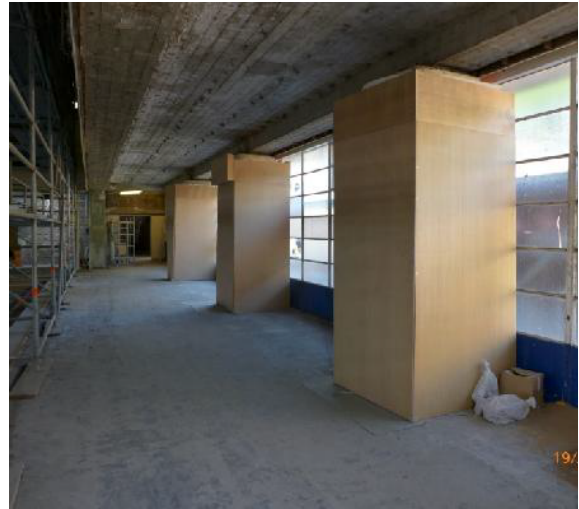
Upper Ground Floor – Protection maintained to the feature columns to the Main Hall.
